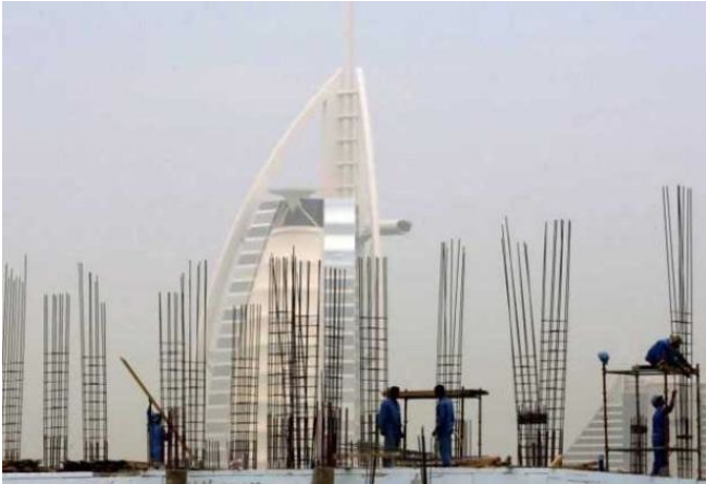
Construction workers in their distinctive blue overalls building the upper floors a new Dubai tower, with the distinctive Burj al-Arab hotel in the background
